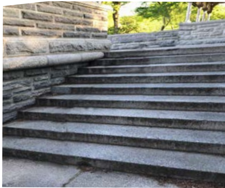
GRANITE TREADS AND CAPSTONES
