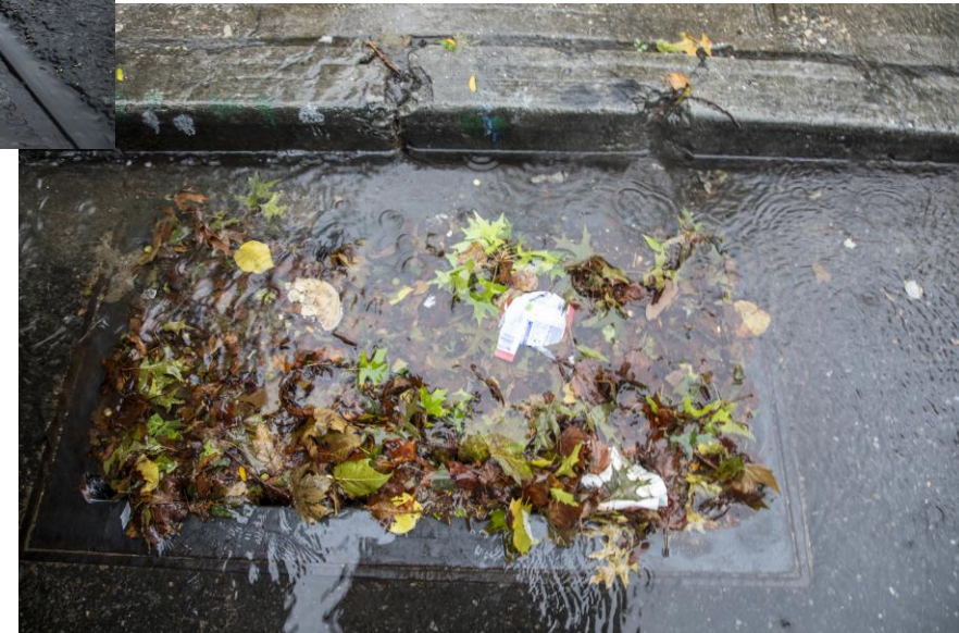
Blocked Catch Basin
