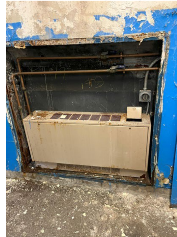
Typical Existing Fan Coil
