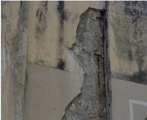
West Wall Concrete Spalls
