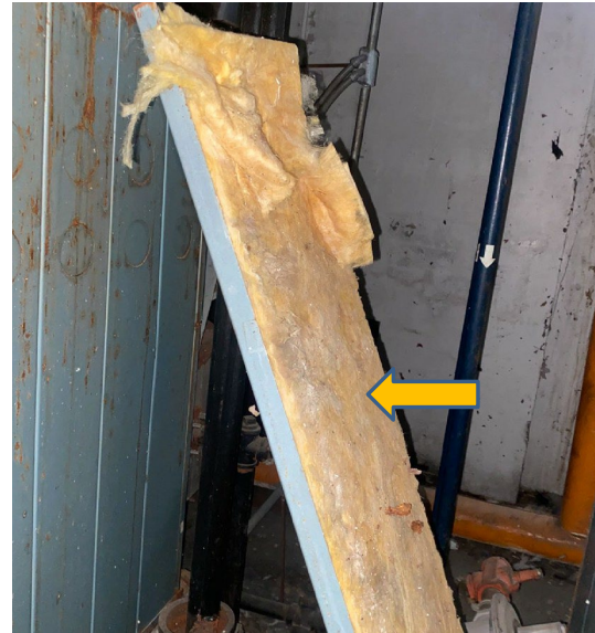
Boiler Cover Insulation
