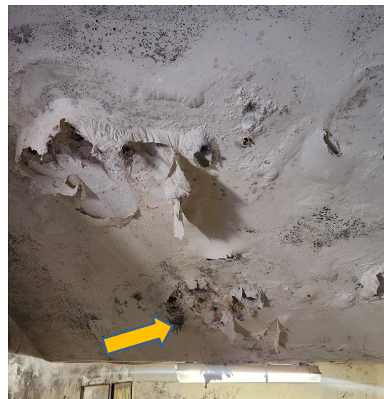
Mold on Interior Walls
