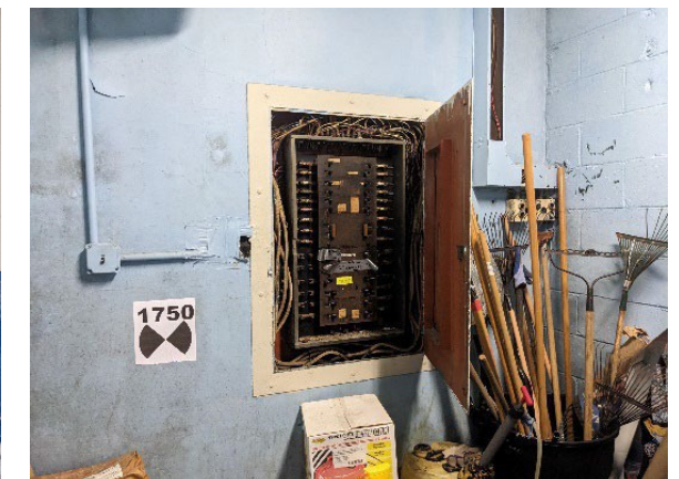
Typical Existing Electrical Panel
