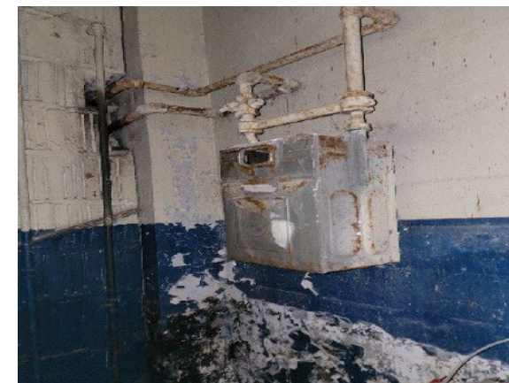
Existing Gas Meter
